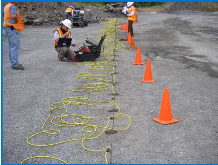
Photo of GeoTrax Survey™ transect (electrode stakes, geophysical cables, and field instruments)
