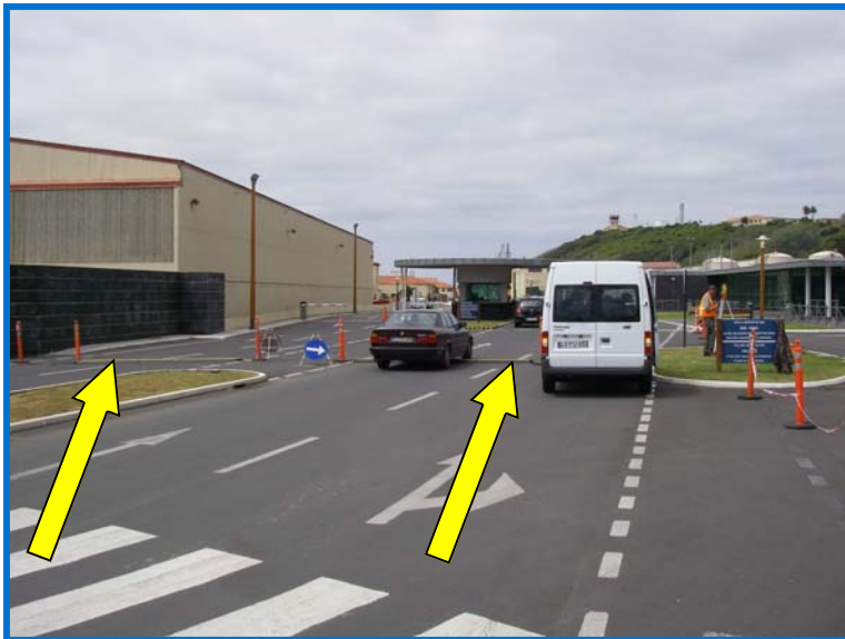
Photo shows traffic ramps over electrodes and cables; allows traffic to flow unimpeded into and out of military base
